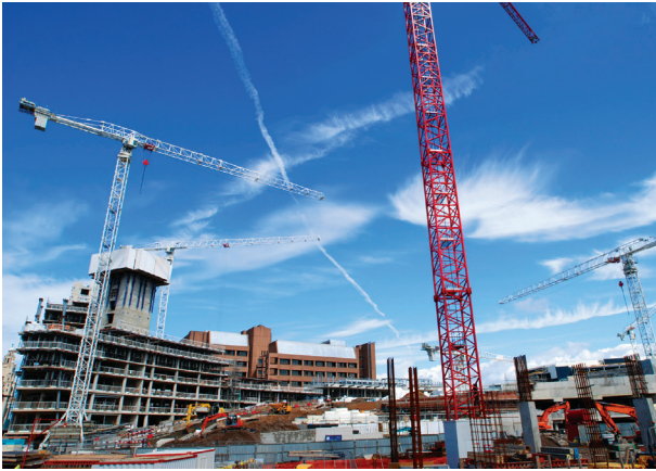
Fig. 1.2 Construction site: BIM enables errors and clashes to be resolved early in the model, rather than later on-site
